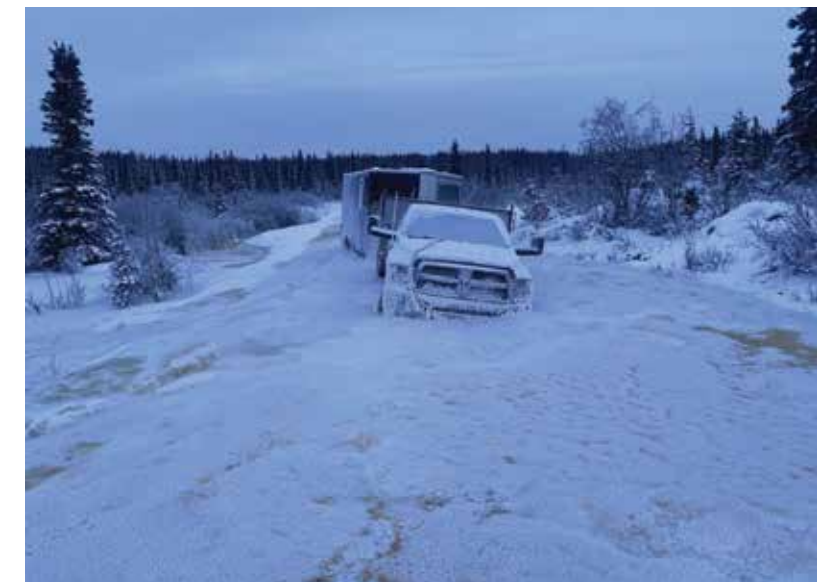
CAFN washed-out road at repair site.
